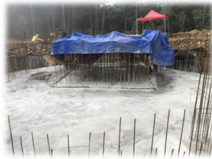
图 3.5: 基墩和建筑物基础浇筑(1.5米以下) Concreting the telescope base pier trough and the foundation of the telescope main building (up to -1.5m of the ground level)
