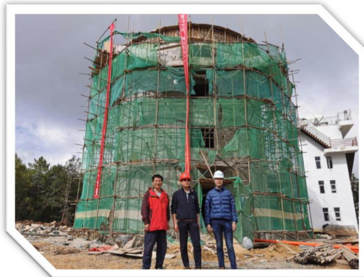
图 3.7: 主体工程封顶 the structural pouring and capping of the telescope main building were completed
