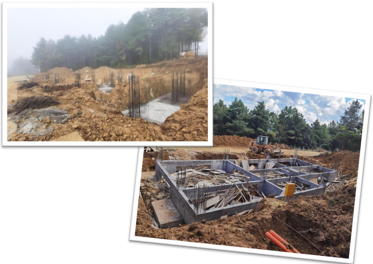
图 3.11: 左: 数据中心基础钢筋绑扎; 右: 数据中心完成基础浇筑 Left: foundation reinforcement binding of the data center; right: foundation pouring of the data center completed
