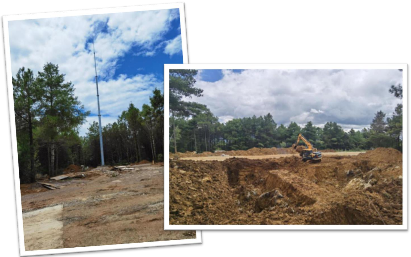
图 3.10: 左: 防雷塔; 右: 数据中心基坑开挖 Left: lightning protection tower; right: foundation pit excavation of the data center
