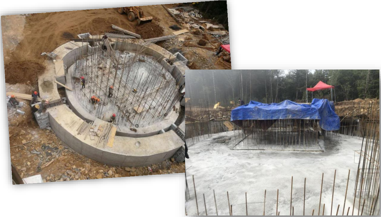
图 3.4: 基墩和建筑物基础浇筑 (至地平-1.5 米) Concreting the telescope base pier trough (up to -1.5m of the ground level)
